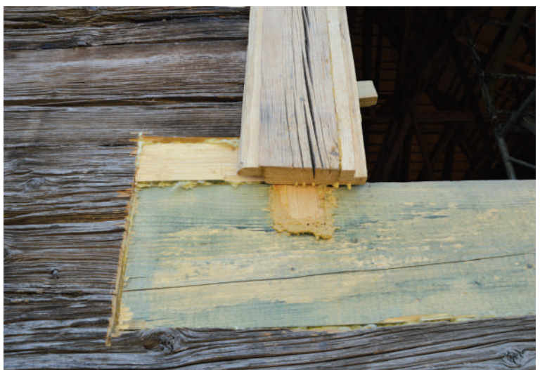
Inappropriate restoration of window frames 2017
